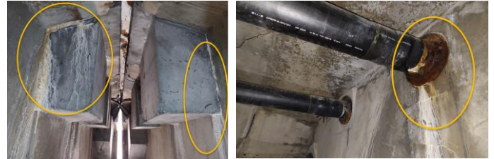
Figure 17. On the left picture, detailed protection anchorages blocks with water circulation. On the right one, evidence of water circulation along the interior prestressing duct.
