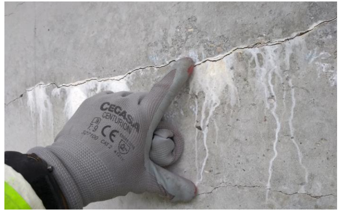
Figure 8. Detailed view of the cracks of the V-Shape beams. Evidence of water circulation and white carbonates spots.
