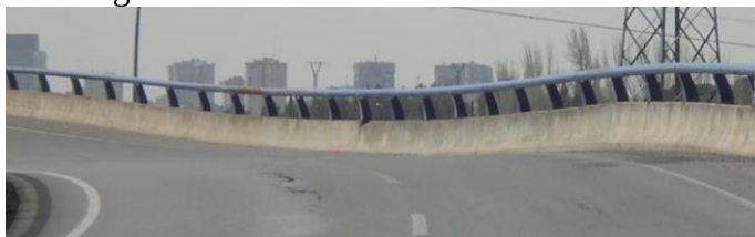
Figure 11. Up to 60 cm deflection in main span. Perfectly visible along the bridge.
