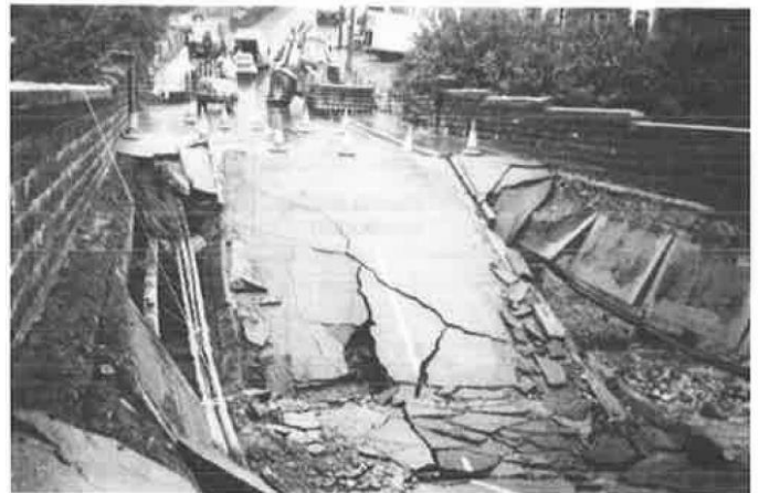
Figure 1. Ynys-y-Gwas Bridge. Segmental Bridge collapsed in Wales. Source: Woodward, R.J. 1989. Collapse of a Segmental Post-Tensioned Concrete Bridge
