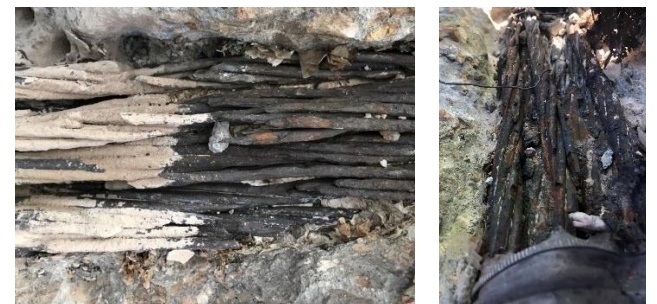
Figure 13. Grouting voids with severe corrosion and broken wires and strands.
