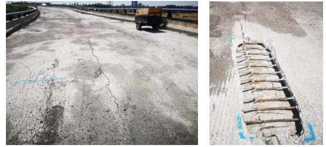
Figure 12. On the left picture, general cracking of the top slab bridge. On the right one, reinforcement bars sectioned along the bigger cracks.
