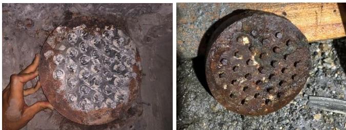
Figure 19. Exterior aspect anchorage block after mortar withdrawal. Different corrosion levels were discovered.
