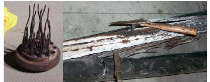
Figure 5. Detailed view of an anchor plate tendon and of a damaged tendon. In both cases, corrosion and grouted problems were detected. Source: Mid-Bay Bridge Post-Tensioning Evaluation
