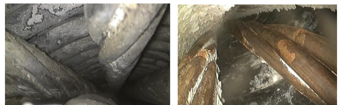
Figure 18. Interior anchorage block inspection by borescope. Significant grout voids detected with strand corrosion. Source: Freyssinet.
