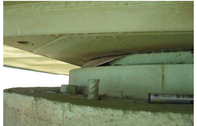
Figure 30. TPFE sheet removal of a POT-bearing.
