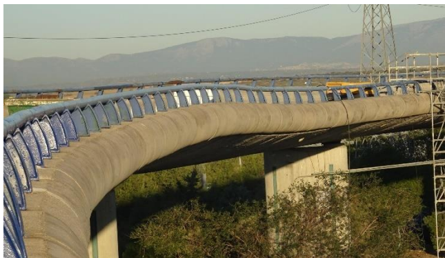
Figure 7a. Serious alterations at the alignment of the overpass located at Colmenar & M40 junction (Madrid).
