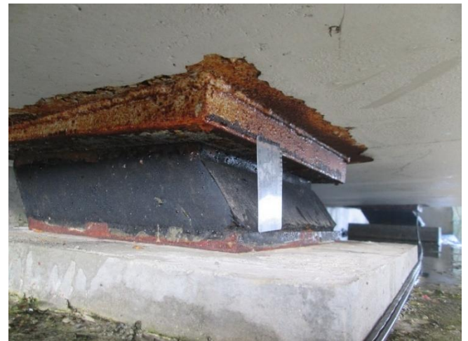
Figure 31. Excessive distortion at elastomeric bearings due to errors in the estimation of imposed deformation.
