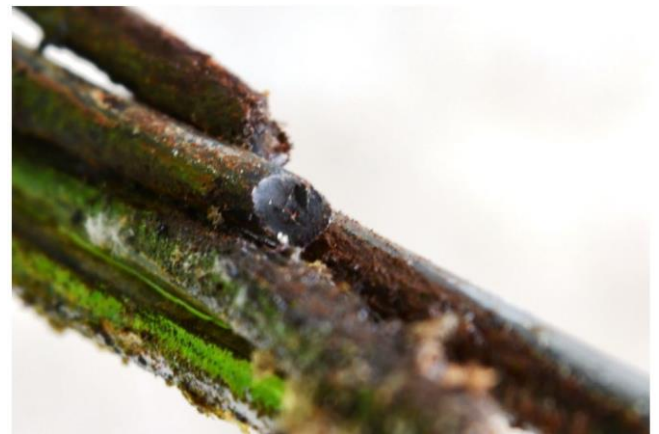
Figure 47. Corrosion detected at some tendons of the Centenary Bridge, 2018
