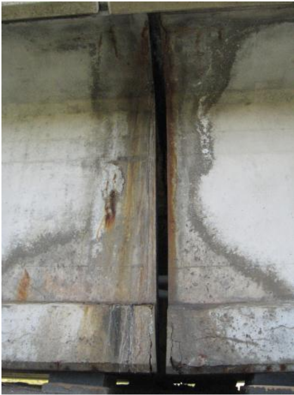
Figure 3. Water leakage through expansion joints.
