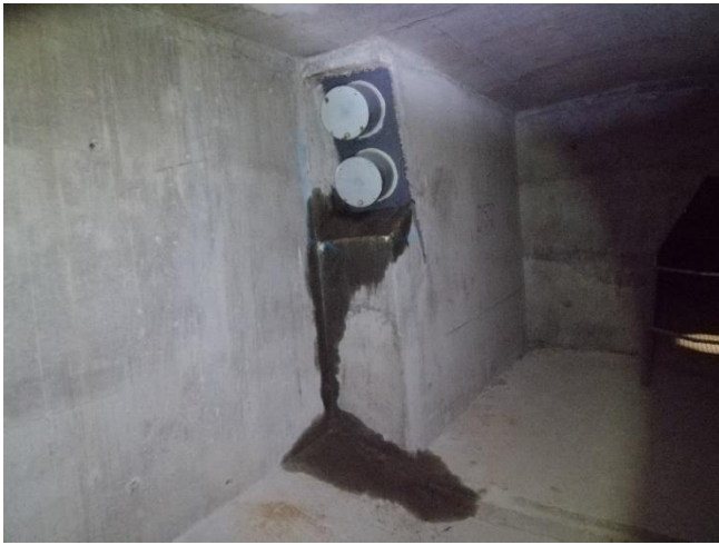
Figure 16. Water leakage through anchor caps of upper cables over piers on a box girder launched railway viaduct.
