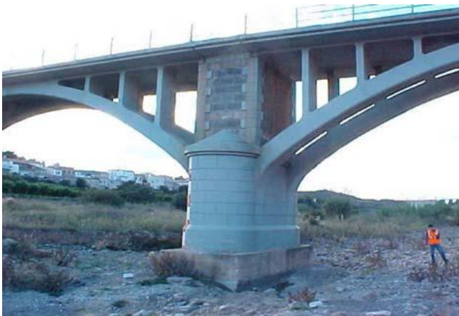
Figure 2. Scouring of foundations.
