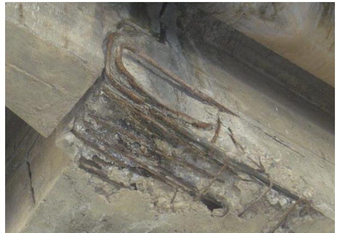
Figure 20. Concrete degradation of spalled corbels with general corrosion at reinforcements
