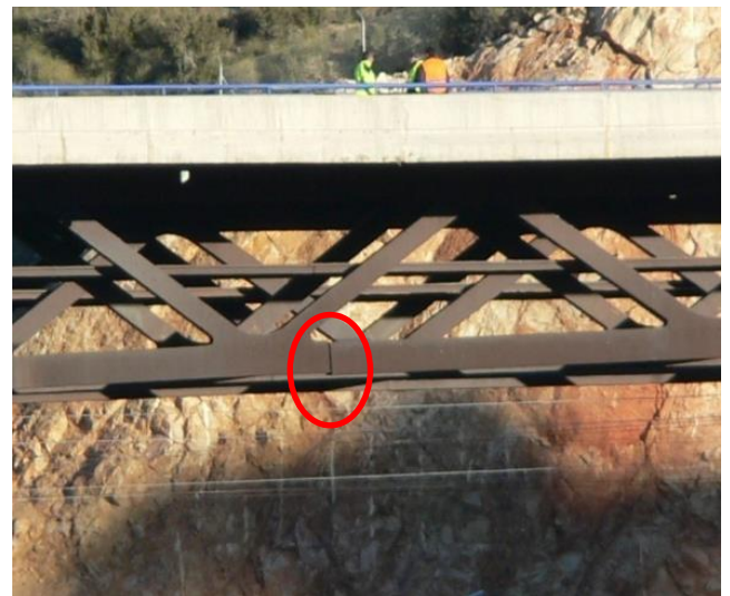
Figure 35. Welding rupture at the truss traction chord.
