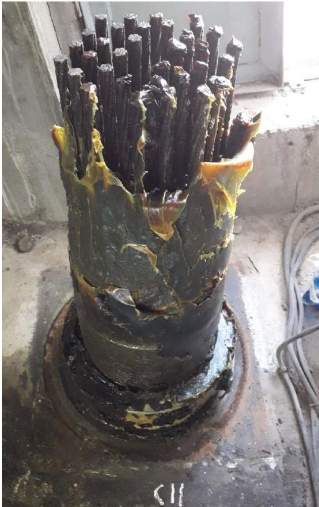
Figure 45. Generalized corrosion at the Alcoy bridge's broken cables (2016).
