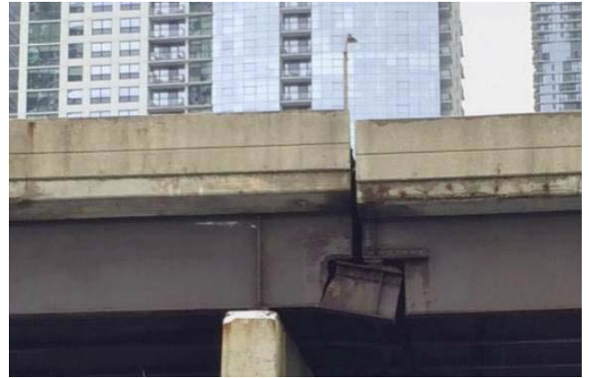
Figure 24. Failure by fatigue of a corbel in a steel bridge, Chicago.
