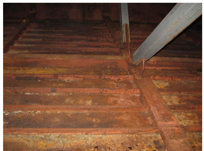
Figure 18. General corrosion at the bottom plates of the Mengibar bridge box girder.
