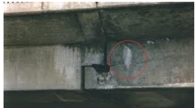
Figure 26. Detail of damages at the Montreal corbel before collapse.
