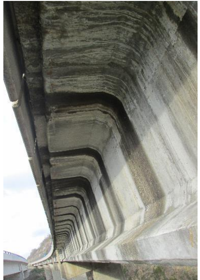
Figure 5. Water filtrations under the platform's side bars.
