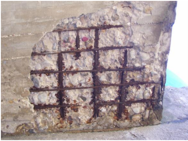
Figure 6. General corrosion due to concrete carbonation.
