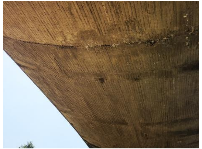
Figure 10. Bottom of deck deterioration due to rainwater drainage failure.
