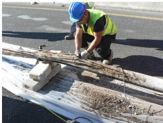
Figure 42. Observed damages in stay-cables with PHD ducts and mortar slurry
