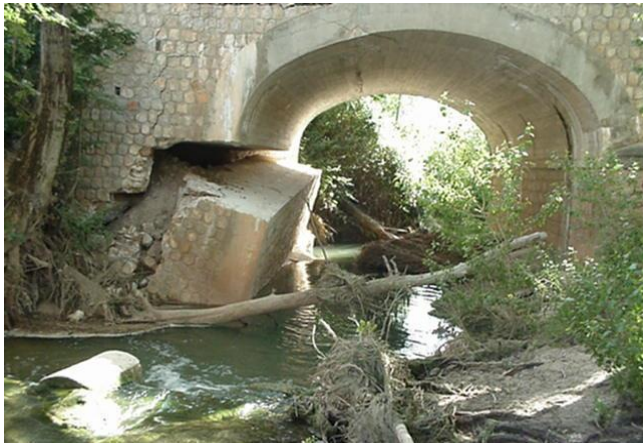
Figure 1. Scouring of foundations.
