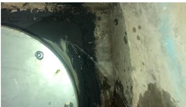
Figure 17. Continuous water flow when loosen some screws of anchors caps.
