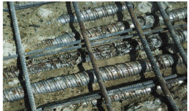
Figure 15. Lack of corrosion protection due to a not-conforming grouting of ducts.
