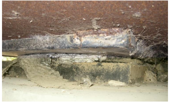
Figure 29. TPFE sheet removal of a POT-bearing.
