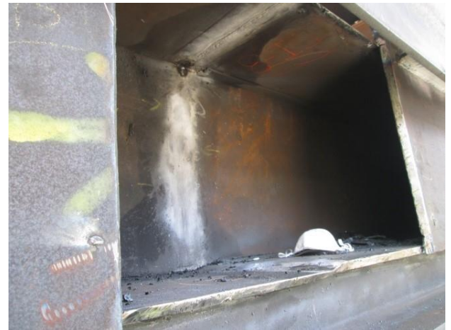
Figures 37a and b. Sections opening for internal inspection and repair (root and backing plate areas).
