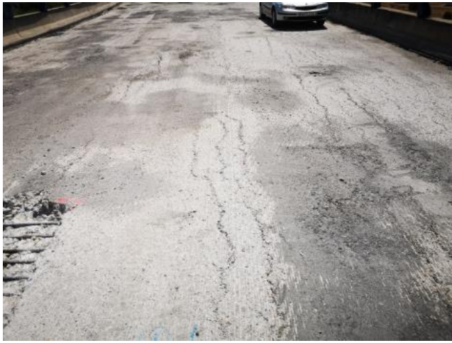
Figure 8b. Cracking and general longitudinal fissures due to alkali-aggregate reaction expansion processes.
