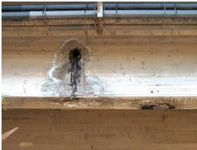
Figure 4. Missing elements in drains.
