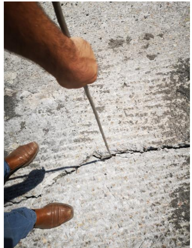
Figure 8a. Cracking and general longitudinal fissures due to alkali-aggregate reaction expansion processes.
