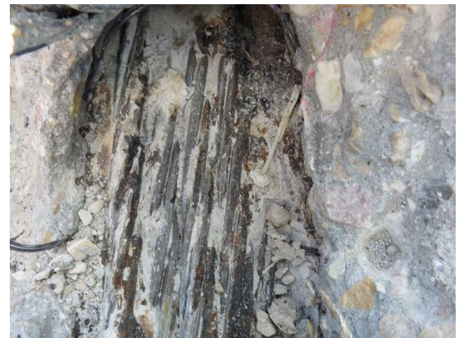
Figure 11. Corrosion of ducts and post-tensioning cables under the action of de-icing salts and a deficient duct injection.
