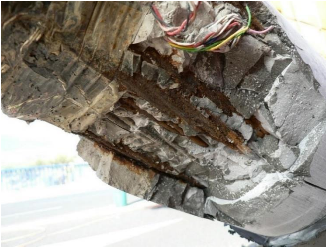
Figure 41. Observed damages in stay-cables with PHD ducts and mortar slurry
