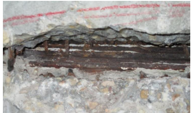
Figure 14. Lack of corrosion protection due to a not-conforming grouting of ducts.
