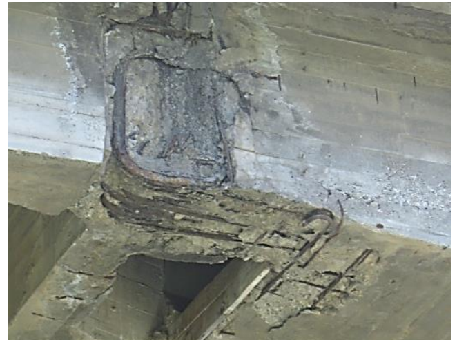
Figure 21. Concrete degradation of spalled corbels with general corrosion at reinforcements
