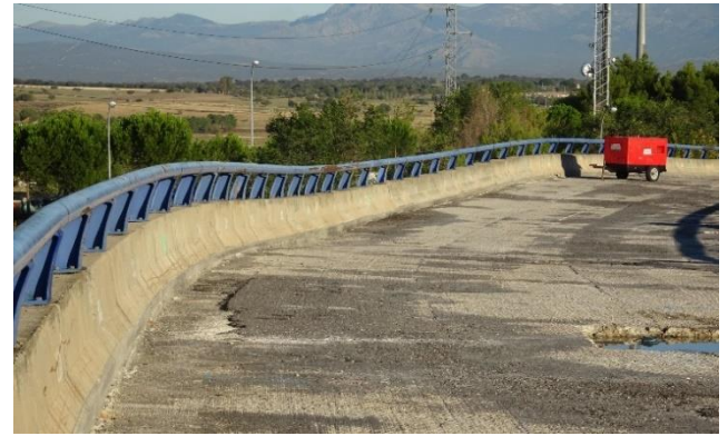
Figure 7b. Serious alterations at the alignment of the overpass located at Colmenar & M40 junction (Madrid).
