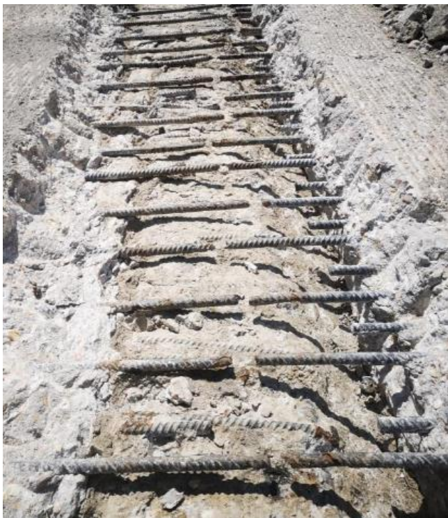
Figure 9. Systematic fractures of the transversal reinforcement due to expansion and corrosion processes under de-icing salts and runoff rainwater.
