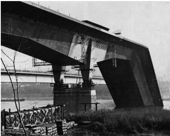
Figure 13. Accident during the cantilever erection of the Koblenz bridge (Germany) 1970
