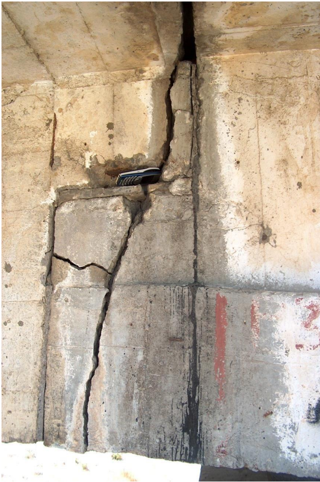
Figure 22. Corbel failure in a concrete bridge.
