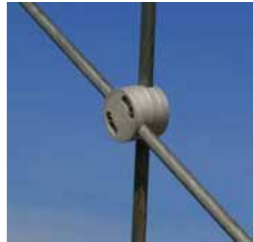
Fig. 27: View of the hanger crossing device.
