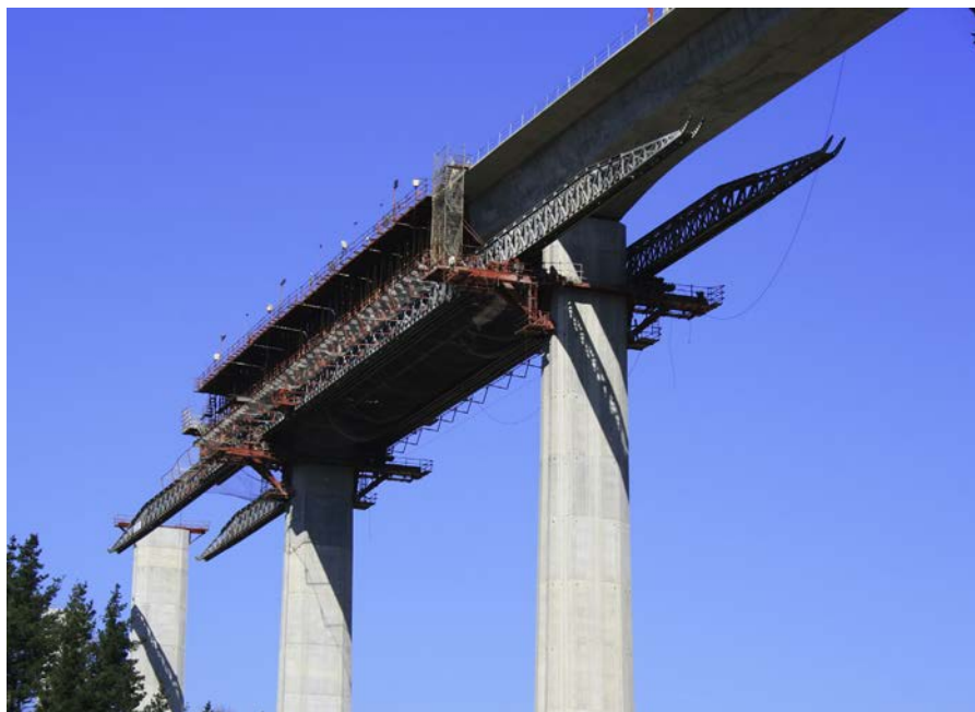
Figure 32. MSS support rings at top of pier.
